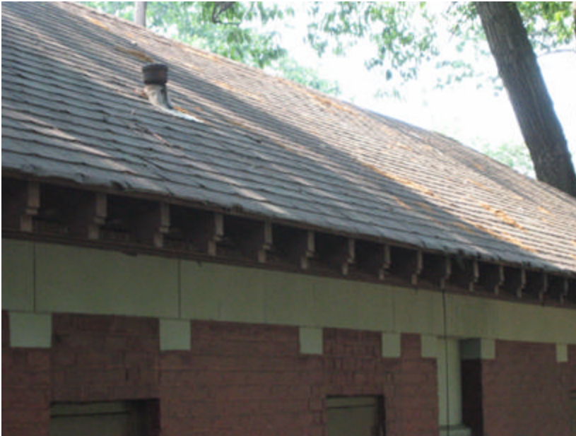
Photo 59 Vertically tooled limestone fascia; note both the brick and wall cap have been painted and the vertical joints are open.
