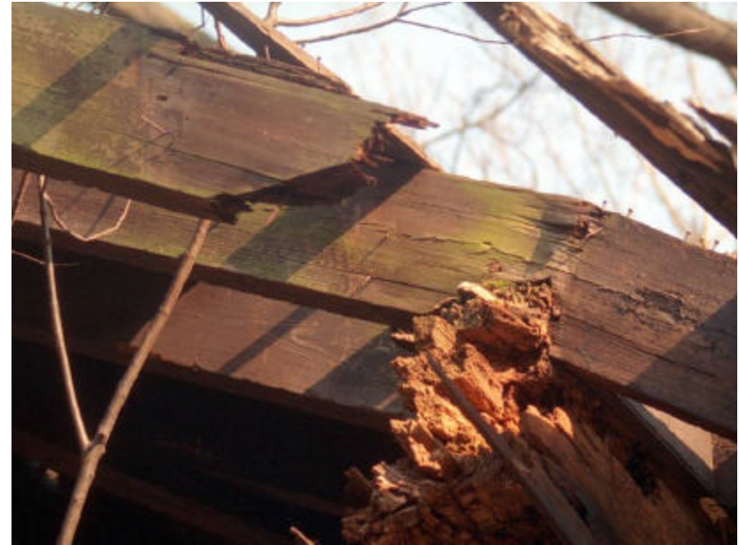
Photo 105 Detail of The Octagon Shelter, column 5.5, showing missing roof support beam, over side 6, and rot and failure of roof rafters.
