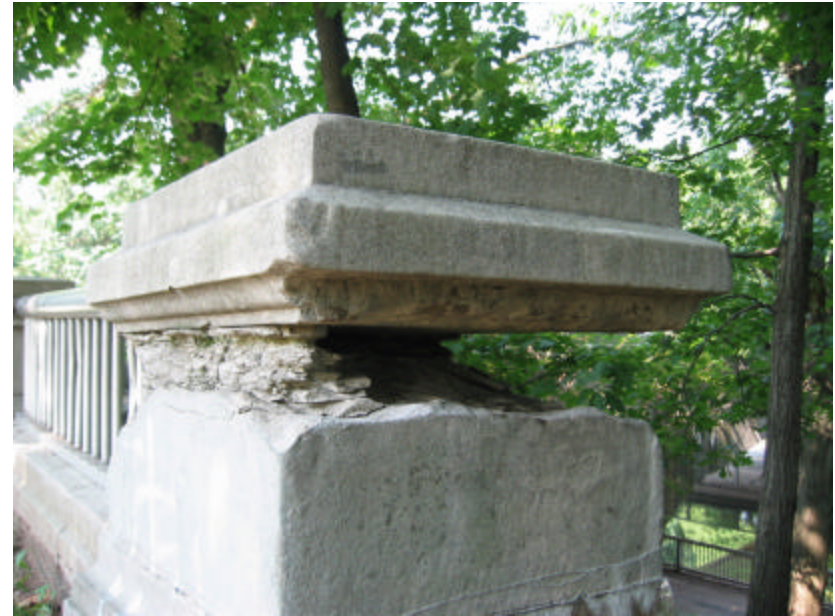
Photo 74 Severe weathering and spalling of concrete on the northeast pedestal; Note that the location is directly below the cap at the bed joint.
