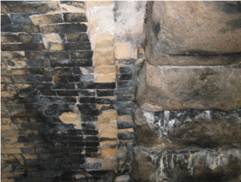
Photo 48 Missing brick from the west side of the underpass; note that this was probably caused by soluble salts leeching down from the road.
