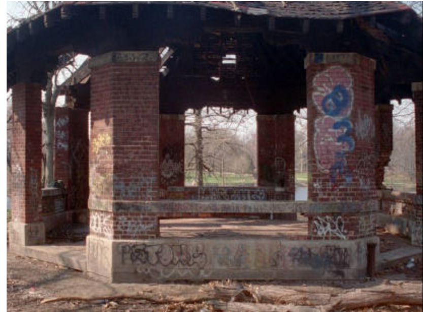
Photo 111 Detail of The Octagon Shelter showing missing brick at side 4 low wall; note that the limestone sill now spans between brick columns.
