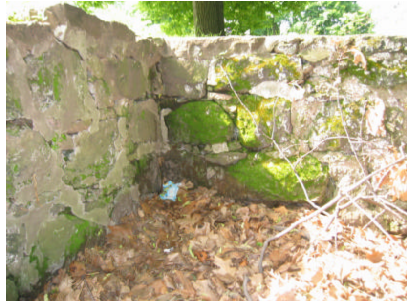
Photo 91 Debris around site; note the biological growth on the wall surface.
