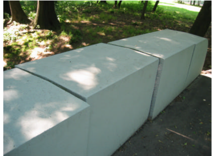
Photo 33 The railing on the east side of Subway 1; note the displacement of the large block of granite and the open vertical and horizontal joints.
