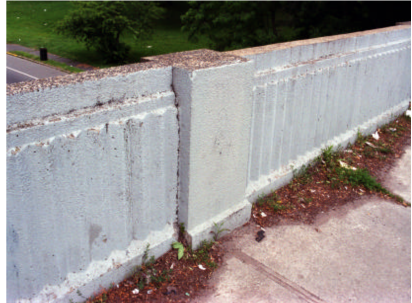
Photo 152 The soiled and painted south parapet wall; note the organic debris at its base.
