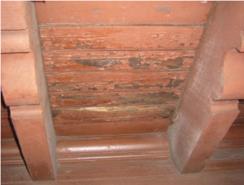
Photo 65 Beaded wood board sheathing on the eastside of the comfort station; note how the wood has rotted.
