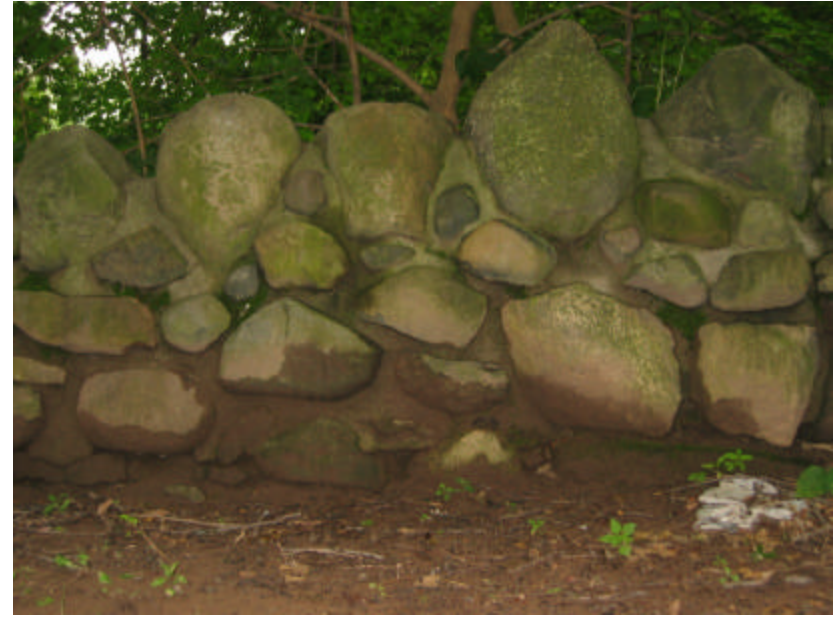
Photo 167 Eroded mortar joints at the base of the south cheek wall; note the soiled fieldstones and mortar.
