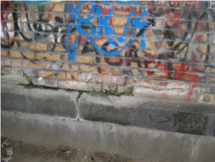
Photo 46 The granite sill along the base of the underpass; note the open joints on the brick and granite.
