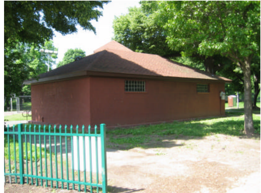
Photo 24 The field house, rear elevation; note that the stucco and roof are in good condition.
