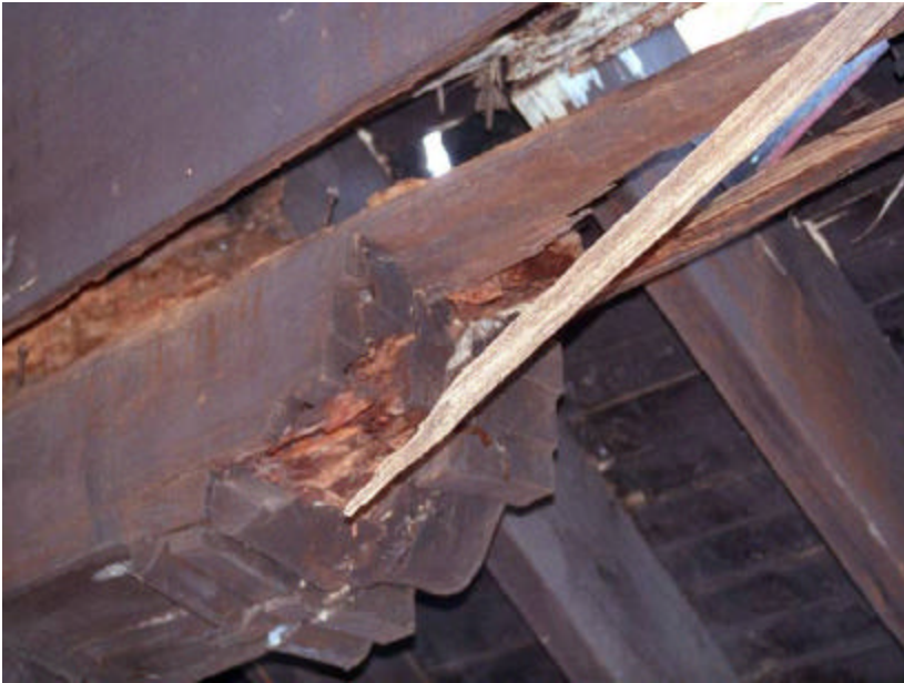
Photo 106 Detail of The Octagon Shelter showing extensive rot of roof support beam; note typical decorative, beam support bracket.
