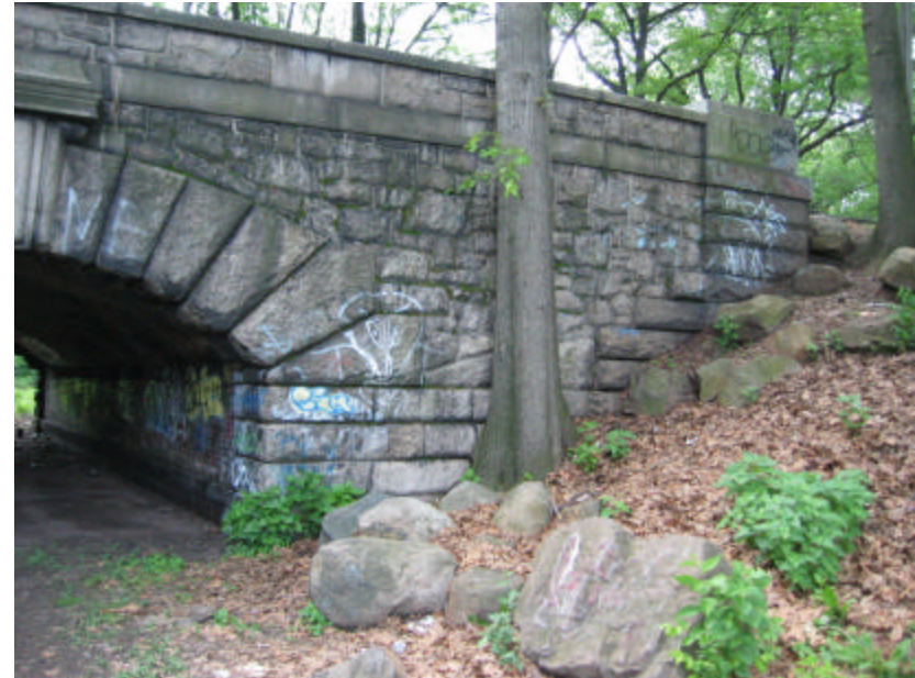
Photo 41 Quarry-faced finishes on the granite; note the broken ashlar pattern of the granite stonework on the vertical face of the underpass.
