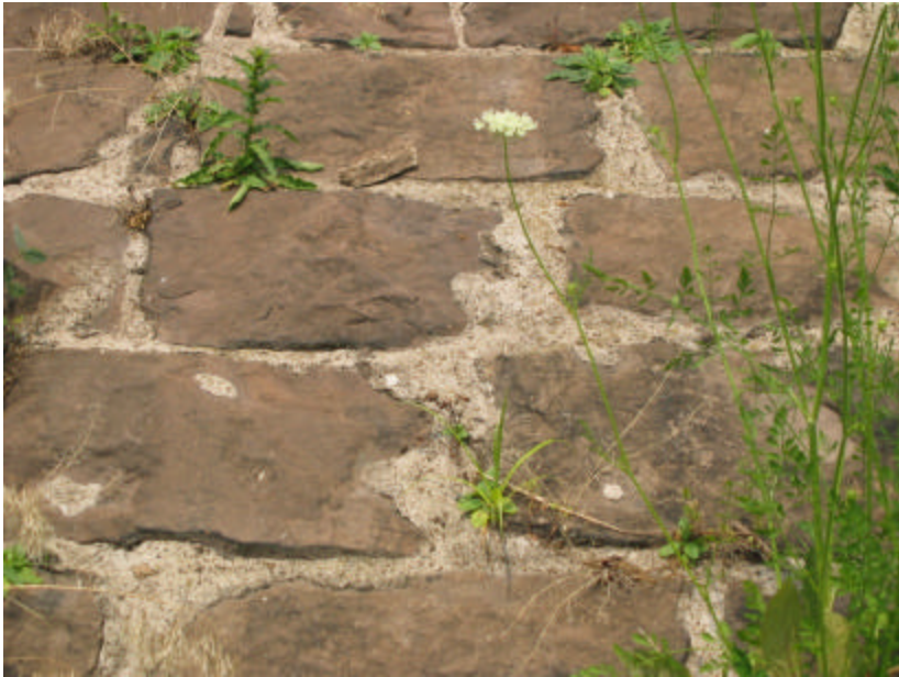
Photo 4 The brownstone blocks that line the walls of the reservoir; note the varying widths of the mortar joints.
