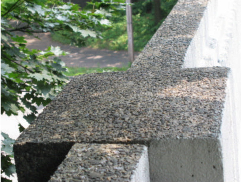
Photo 153 The rough, unpainted concrete surface on the top of the parapet wall; note the open horizontal joint between the post and wall.
