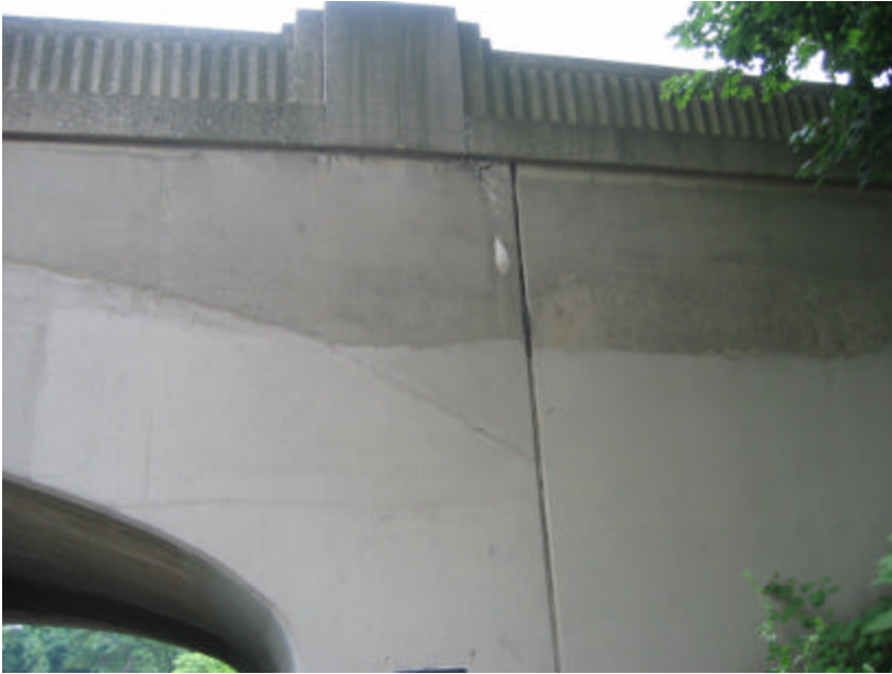
Photo 155 The north side of the bridge is in good condition but there is some cracking, spalling and soiling; note the non-matching paint.
