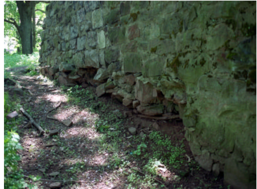
Photo 99 Large amounts of stone missing from the base at the north side of the wall; note that the wall has cracked here because the wall structure is unstable.
