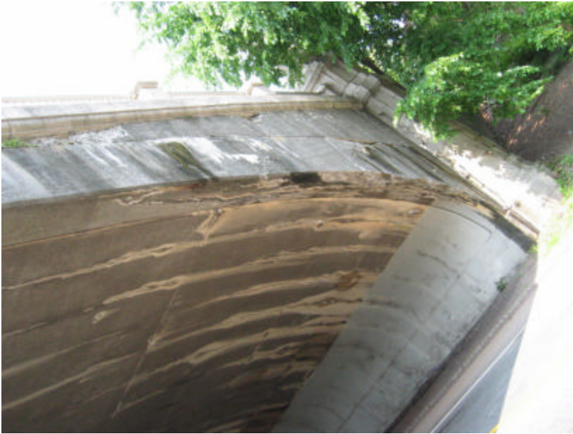
Photo 79 The north side of the bridge; note the heavily soiled surface, cracking and spalling.
