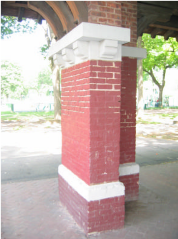
Photo 15 One of the "L" columns at the southwest corner; note the brick and limestone have been painted and that the mortar is deeply eroded.
