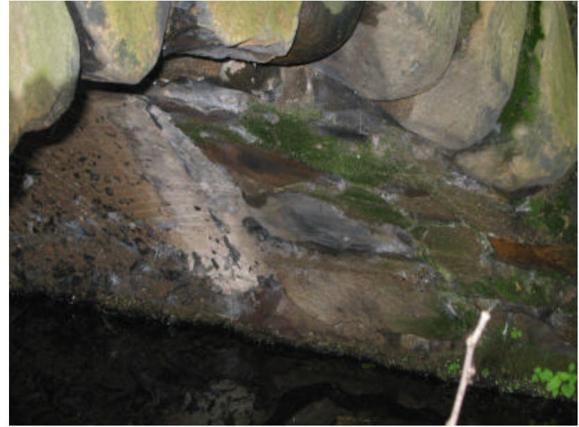
Photo 165 The underside of the fieldstone and concrete arch on the south side of the bridge; note the moss and efflorescence on the surface caused by water migration from above.
