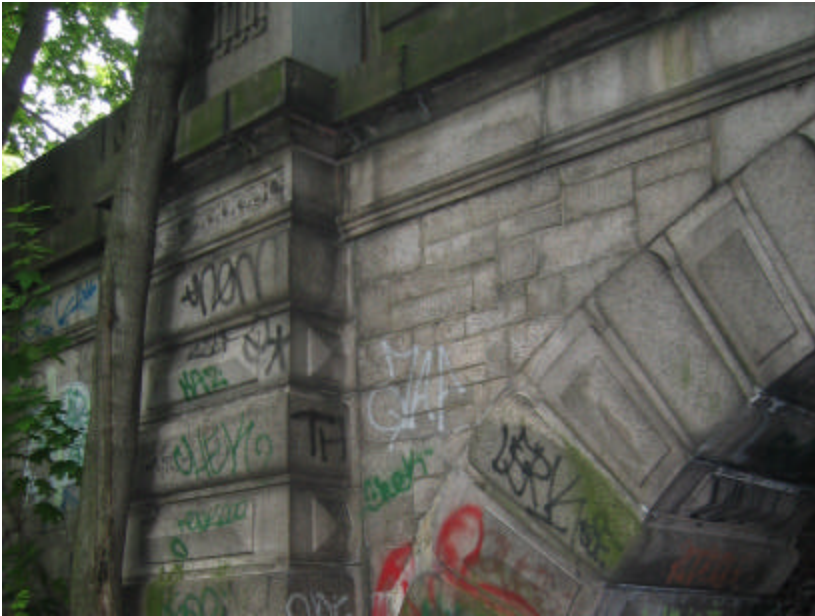
Photo 30 The face of the west side of Subway 1; note the random ashlar pattern of the granite stonework on the vertical face of the underpass and the graffiti covering the surface.
