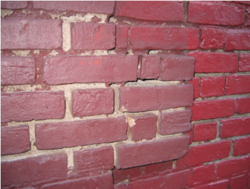
Photo 63 Detail of bricks on the east wall of the building; note that the mortar has almost fully eroded between the bricks.
