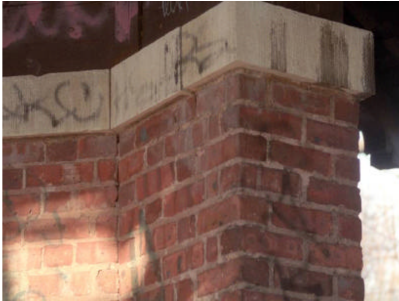
Photo 118 Detail of The Octagon Shelter showing limestone column caps above brick column No. 2.5; note that the higher brick mortar joints are in better condition than those closer to the sill.
