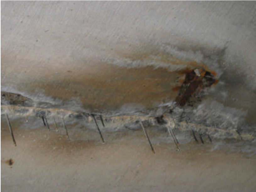
Photo 149 Efflorescence and mineral deposits forming stalactites on the underside of the bridge; note the reddish-brown discoloration caused by rusting steel.
