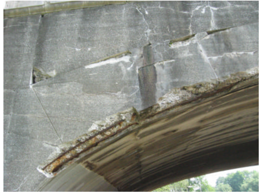
Photo 80 The southwest face of the bridge; note the rusted, exposed steel reinforcing in the concrete.
