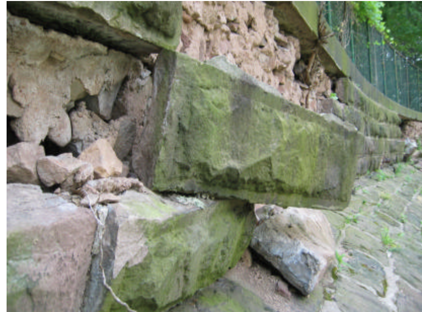
Photo 9 Spalled and missing stone from the wall; note that there is a significant amount of stone missing from this area and the block in the photograph is ready to fall.
