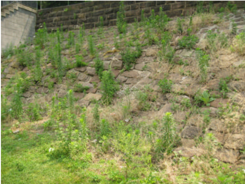
Photo 8 The sloped wall near the concrete staircase; note how the brownstone has been significantly displaced, causing the surface to be extremely uneven.
