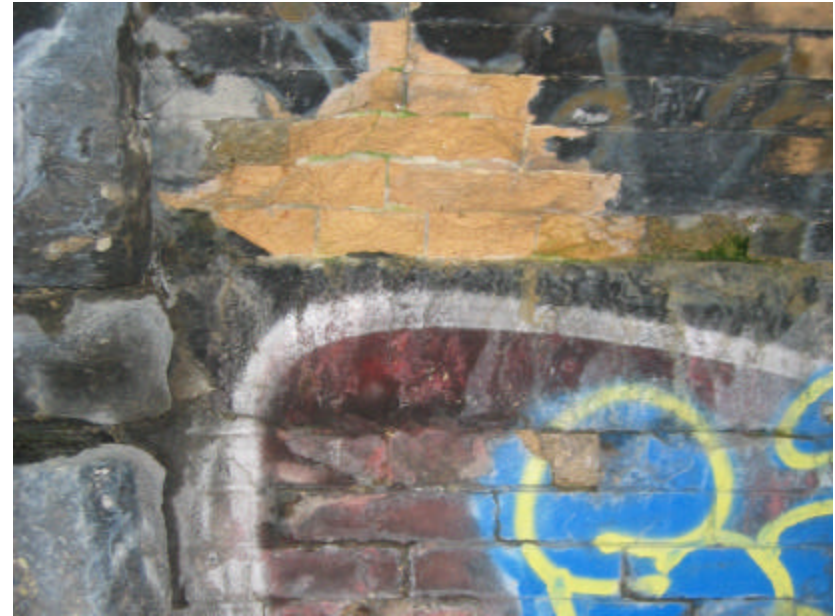
Photo 47 Spalling of brick caused by freeze-thaw cycles; note the staining and Efflorescence.
