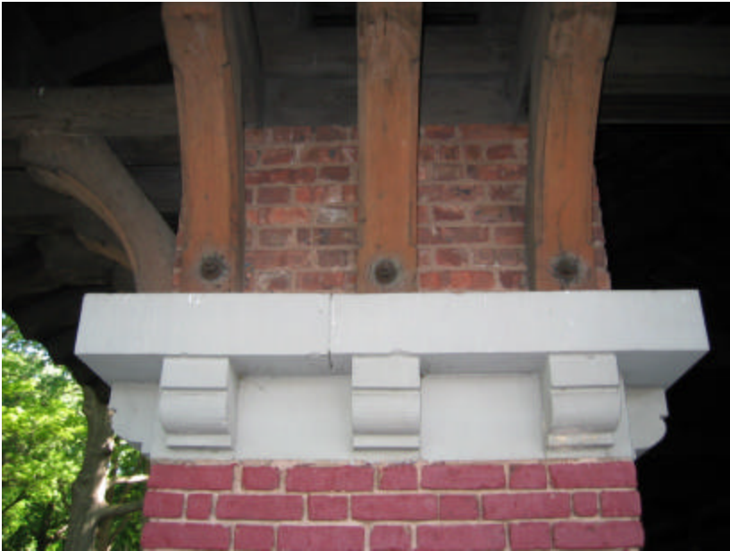
Photo 17 The limestone block and brackets above one of the "L" columns; note the staining and cracking of the wooden brackets.
