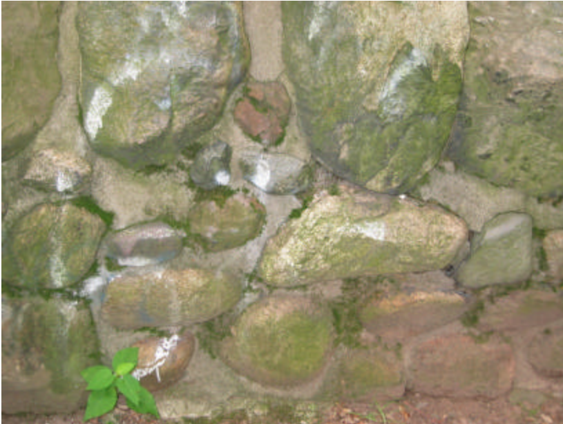
Photo 162 Graffiti and organic growth on the surface of the fieldstones and mortar joints.
