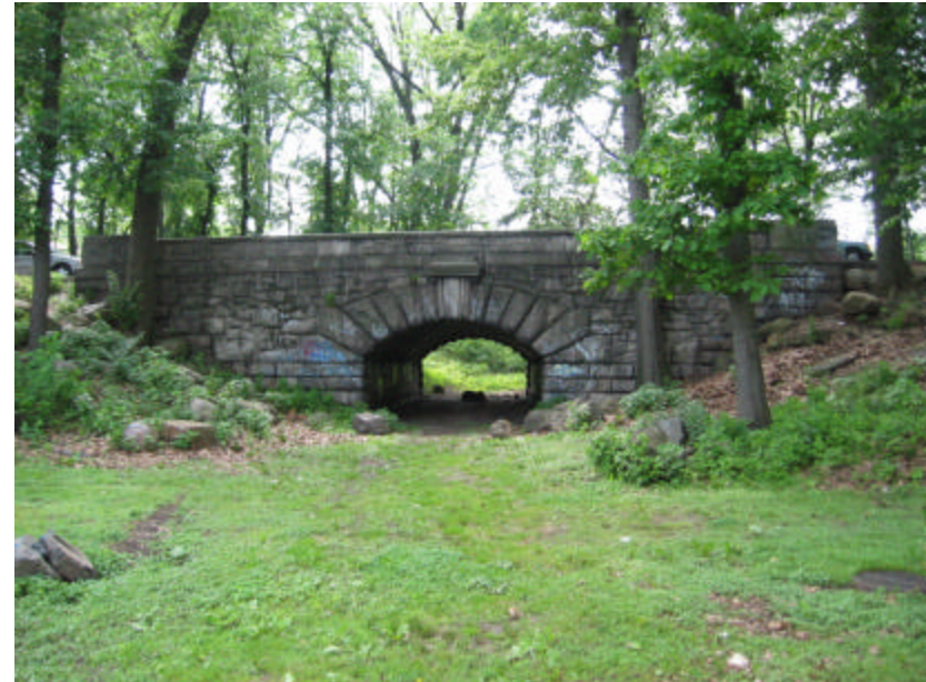
Photo 39 Subway 2 view to the west; note the segmental arch construction and the rustic finish on all the granite stonework.
