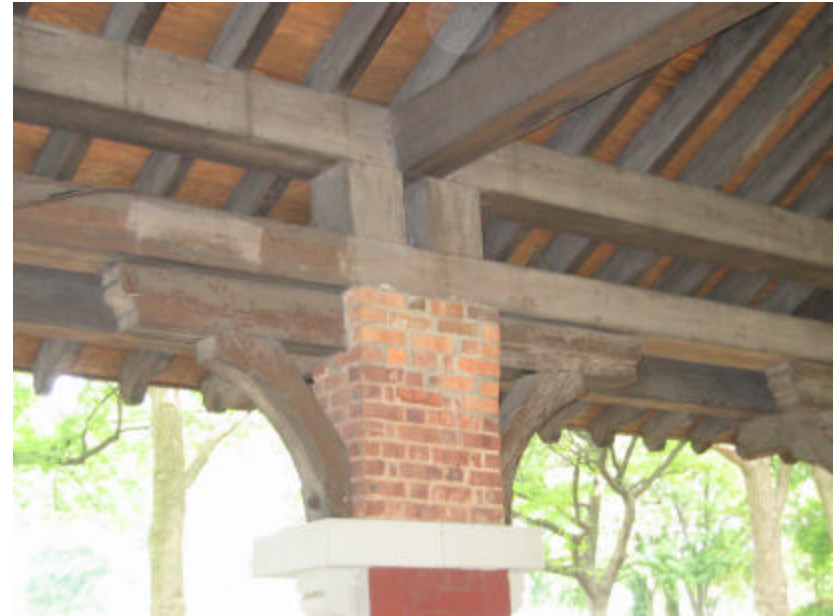
Photo 20 The heavy timber framing that supports the roof structure; note the unpainted bricks above the limestone block.
