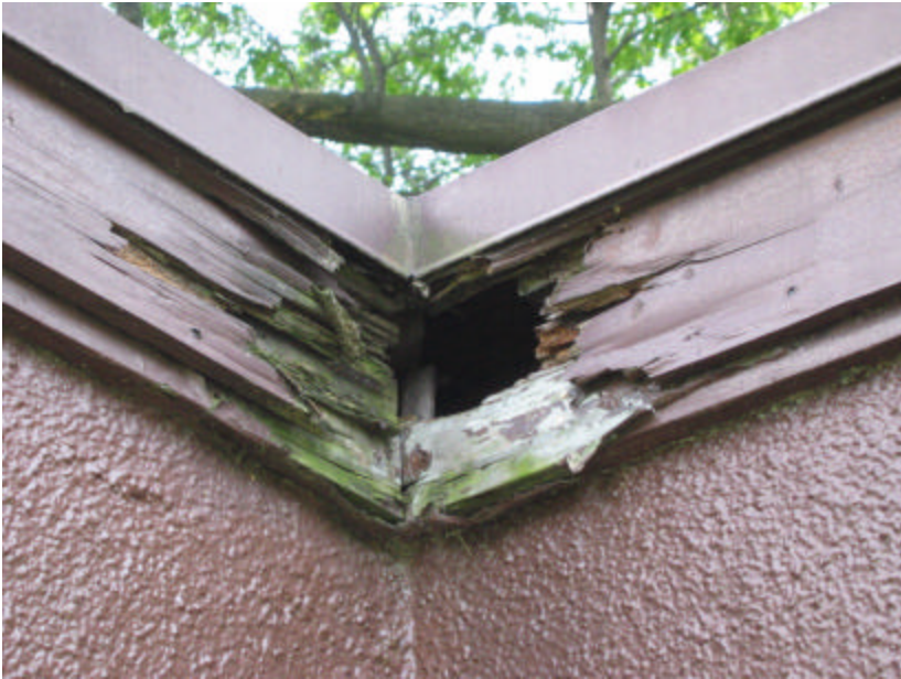
Photo 56 Damage to the wood cornice of the south restroom; note that there is a hole in the wall and that wood has rotted considerably.
