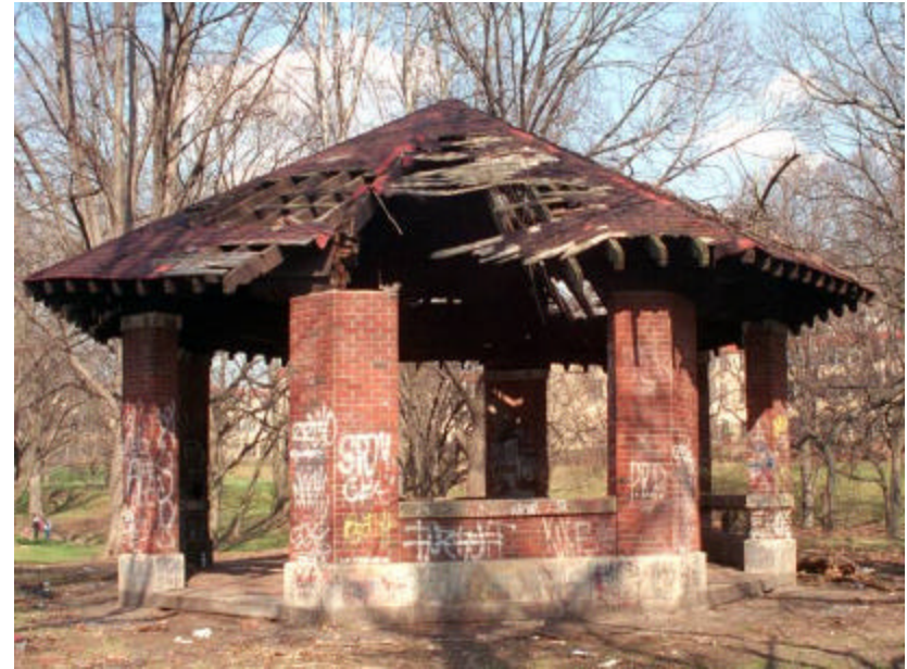
Photo 103 View of The Octagon Shelter from the southwest (side 6 closest); note absence of beams which support wood roof structure.
