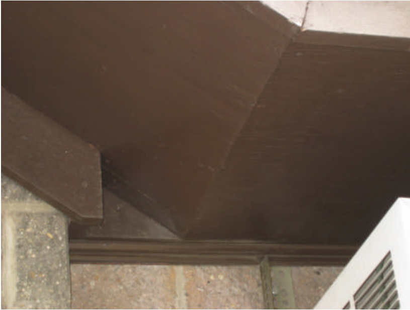
Photo 128 The painted plywood soffit of the cornice; note that it is in good condition with only slight wear.
