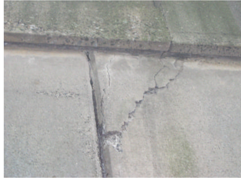
Photo 156 Concrete cracking on the north spandrel wall; note that the cracking appears below the parapet wall and next to an expansion joint.
