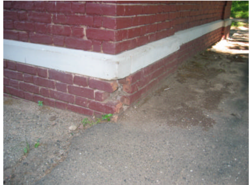
Photo 62 Missing brick from the northeast corner of the comfort station; note that all the brickwork needs to be repointed.
