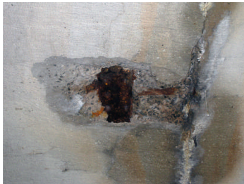
Photo 148 An area of spalling concrete and efflorescence on the underside of the bridge; note the rusted steel beam and rivets.
