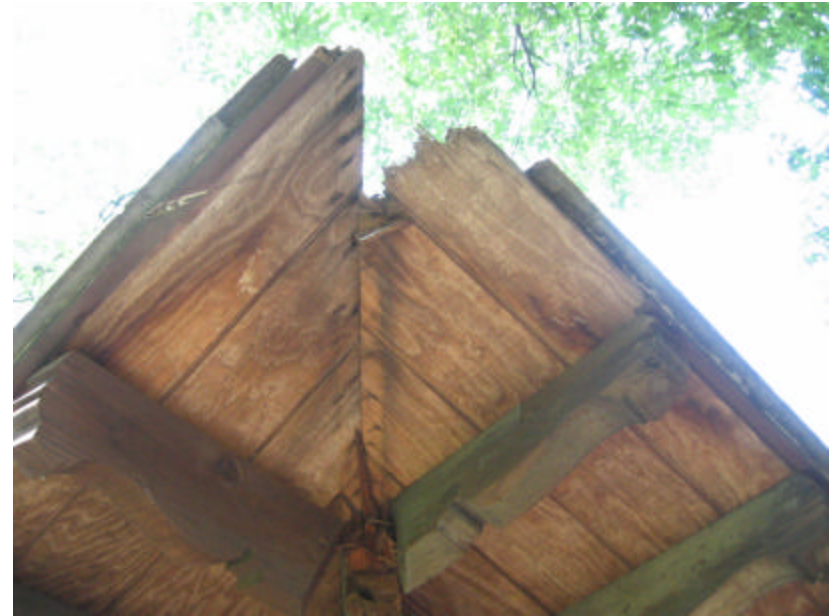
Photo 22 Damage to eaves and roofing; note that one of the eave supports is missing.
