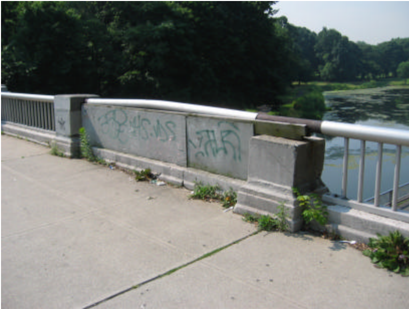
Photo 77 These two posts are severely damaged and missing their caps; note the missing railing as well.
