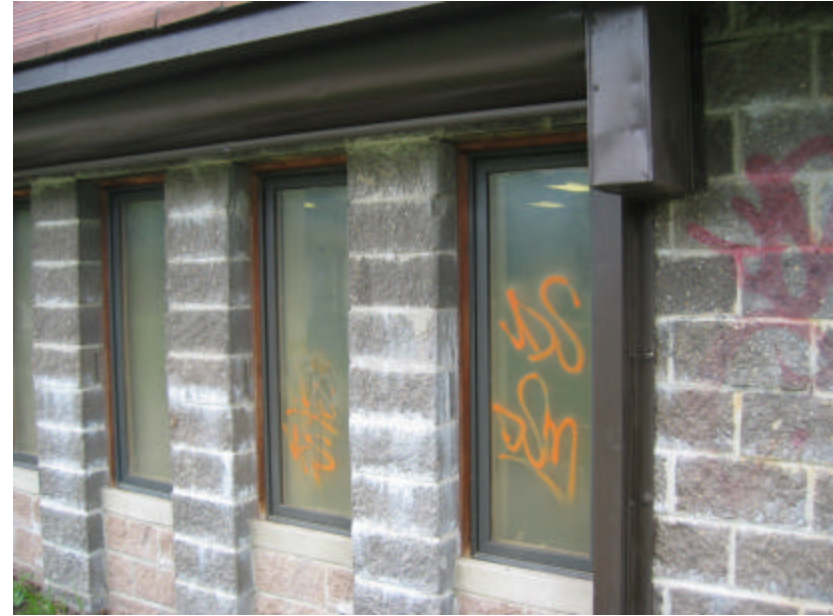
Photo 131 Three of the windows on the south façade; note the fogged plexiglas and the graffiti.
