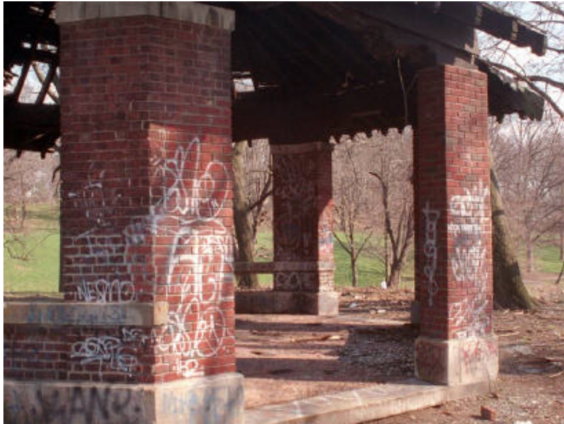
Photo 112 Detail of The Octagon Shelter from the west showing reconstructed brick columns, (No. 7.5 to the left); note that the limestone sills were altered, and do not divide the column as originally constructed.
