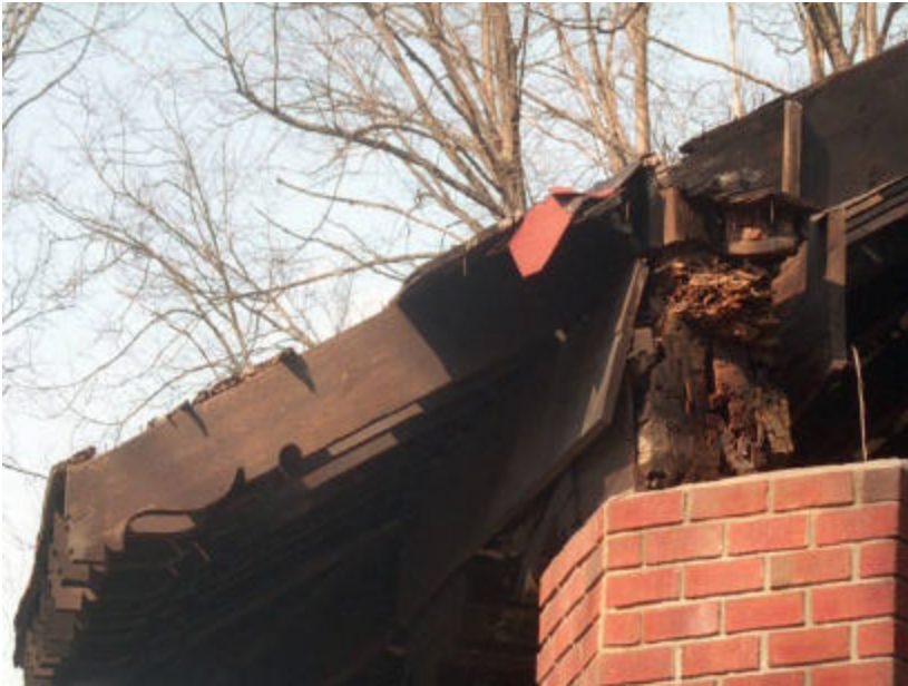
Photo 104 Detail of The Octagon Shelter, column 6.5, of missing roof support beam showing rot of remaining beam as well rot at adjacent roof rafters; note that the roof rafters extend over the beam as decorative eave supports
