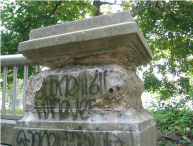
Photo 75 Severe weathering and spalling of concrete on the southeast pedestal; note that the damage has occurred in the same place.
