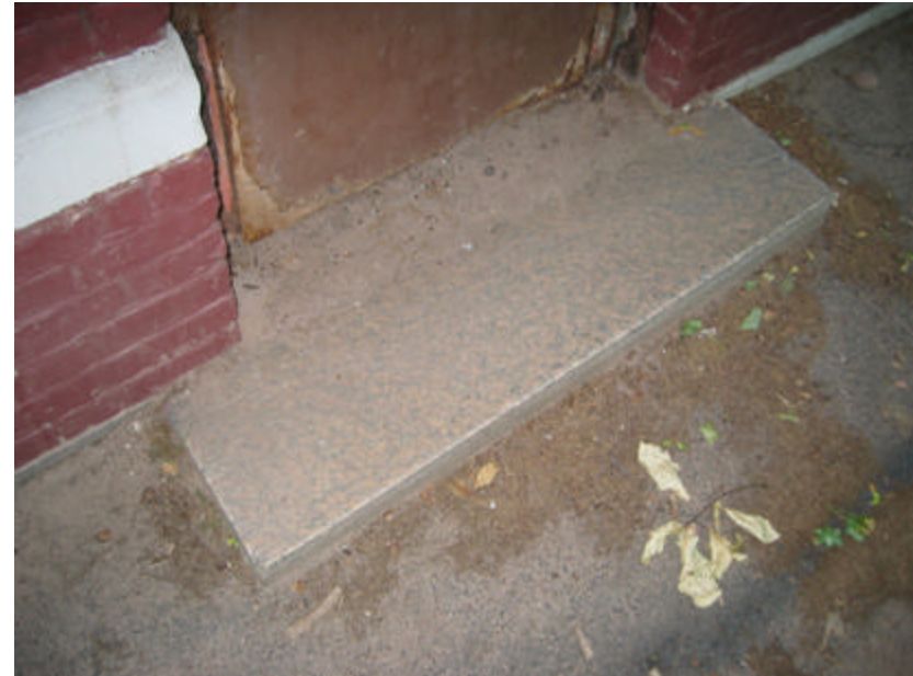
Photo 60 Granite stoop at one of the original entrances to the comfort station; note the damage to the metal clad wood door and the wear to the painted limestone trim.
