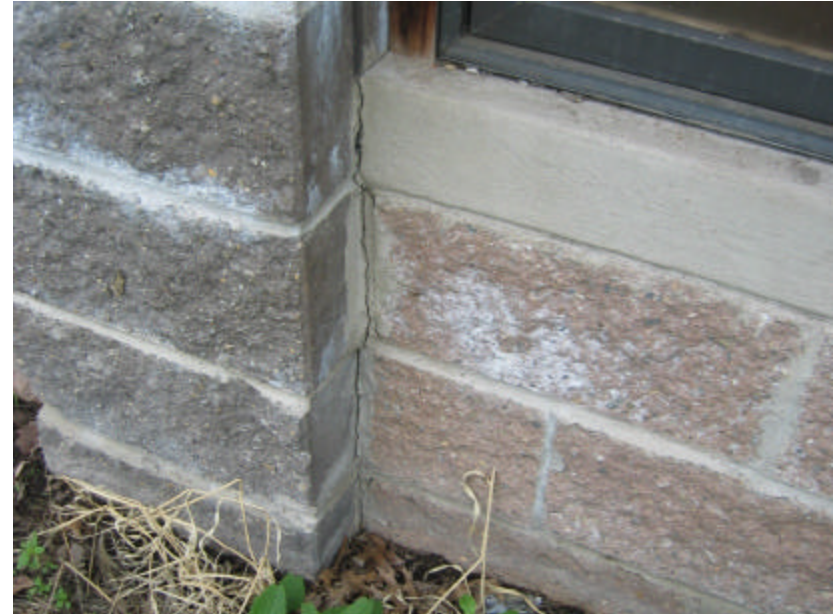
Photo 135 Vertical cracking from a windowsill to the base of the building along one of the mortar joints.
