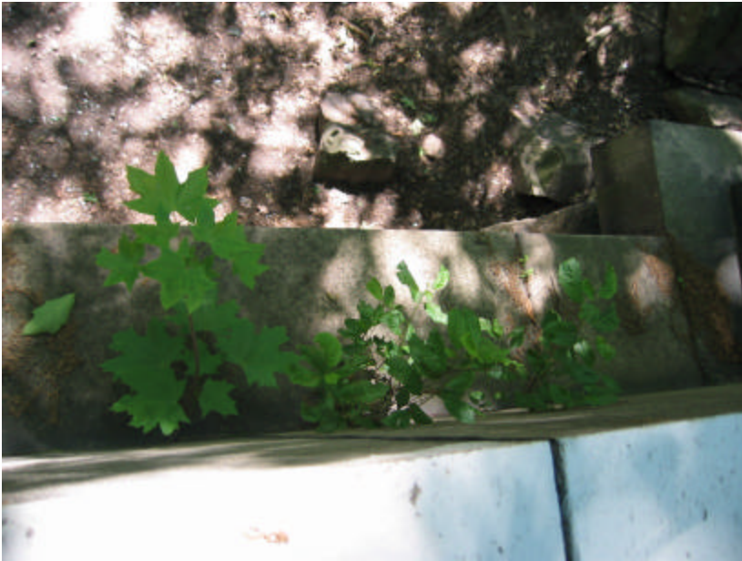
Photo 34 Plants growing out of the cracks in the lintel course below the railing.
