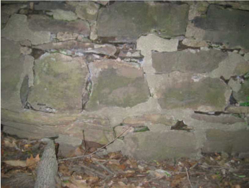
Photo 92 Remedial patching of the masonry; note the patching in most places is poor and that the wall should be entirely repointed.
