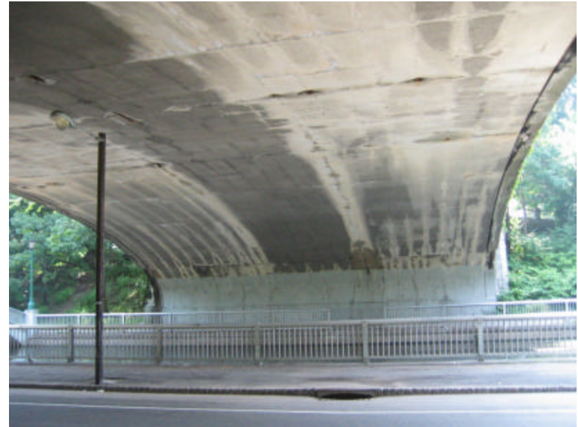
Photo 70 Soiling and spalling on the underside of the bridge; note both the vertical and horizontal cracking.
