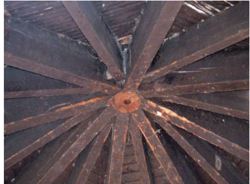
Photo 107 Detail of The Octagon Shelter roof structure; each of 8 major rafters rests on a column and smaller rafters (7 on each side) frame into the major rafters.
