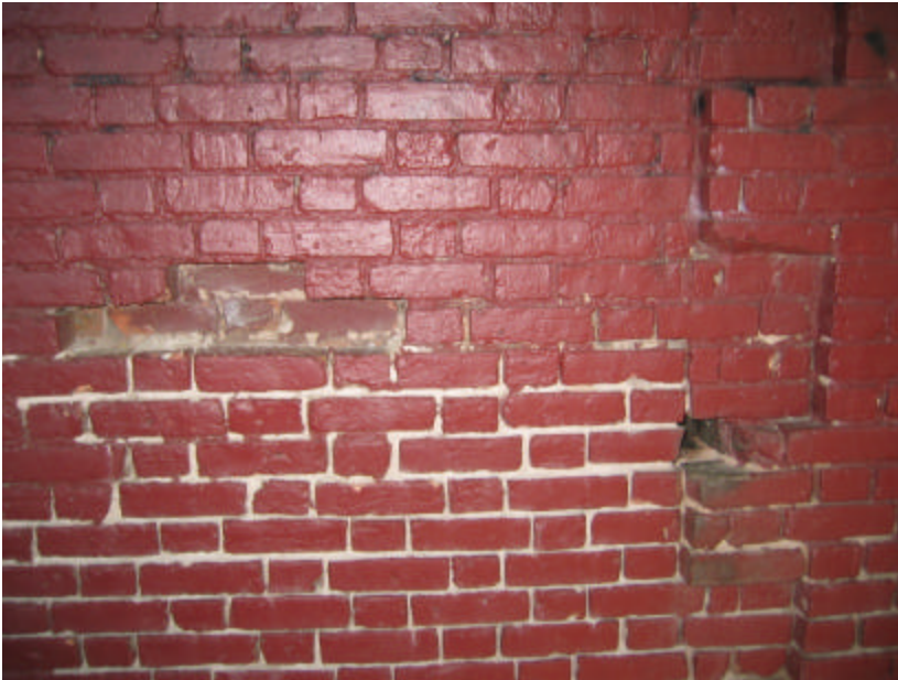
Photo 61 Severely eroded mortar joints and missing brick from the northwest corner of the comfort station; note the brick quoins on the right side of the image.
