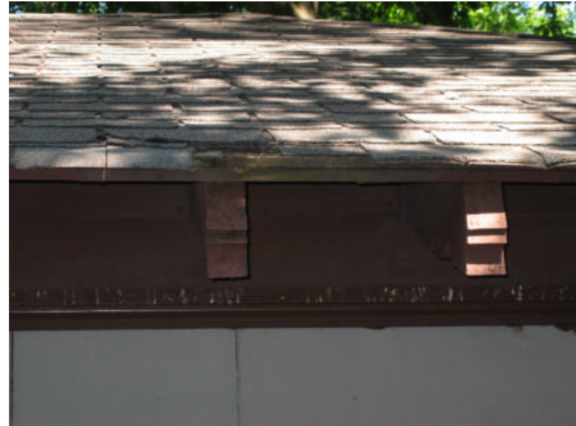
Photo 66 Rotted and broken roof sheathing; note that the asphalt roof tile has failed here and on most edges of the building.
