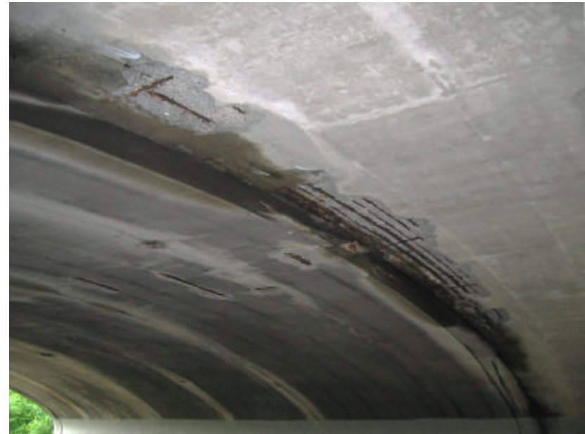
Photo 144 The underside of the bridge; note the soiled concrete and exposed, rusted steel reinforcing.
