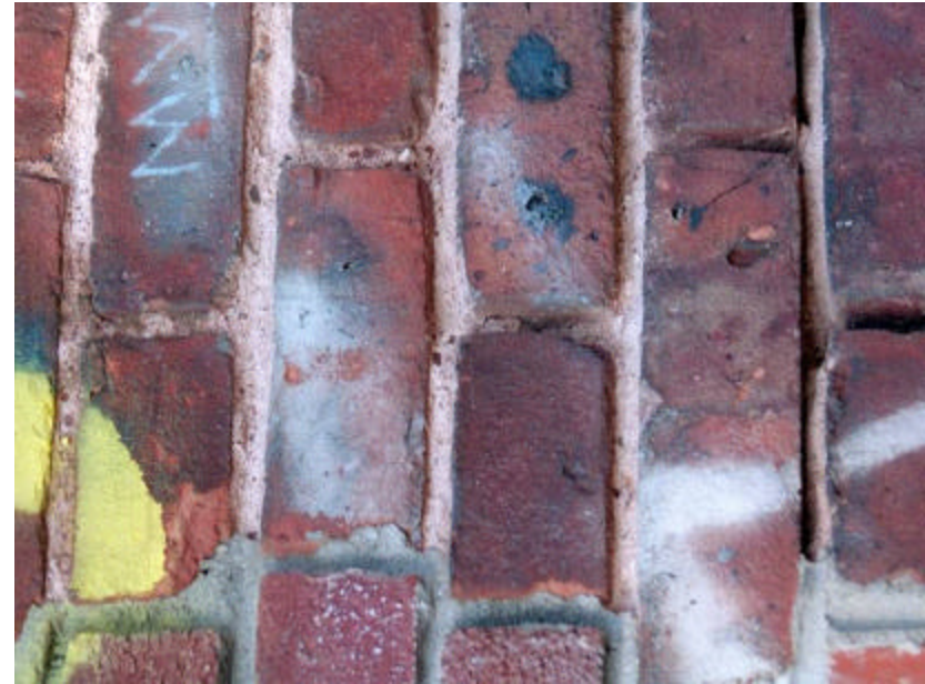
Photo 119 Detail of The Octagon Shelter showing typical, original, eroded, tinted brick mortar joints; note non-matching gray mortar.
