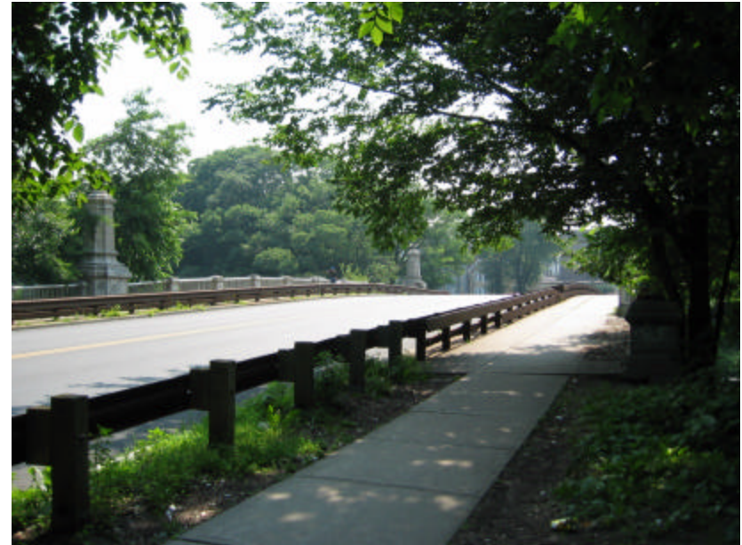
Photo 68 Park Avenue going over the bridge; note the rusted steel vehicular guardrail on both side of the road.
