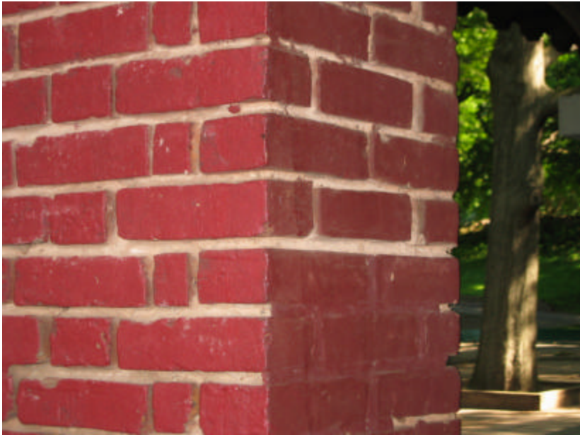
Photo 19 Deeply eroded joints in one of the columns; note that the bottom right portion has been patched and the mortar joints painted over.
