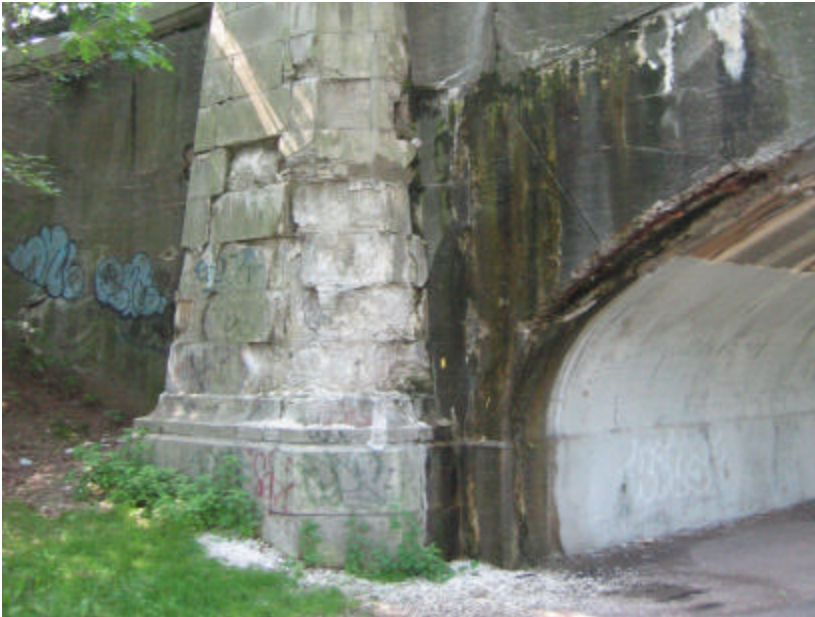
Photo 69 Cracked and spalling concrete on the northeast buttress; note the graffiti, efflorescence and green and black biological growth.
