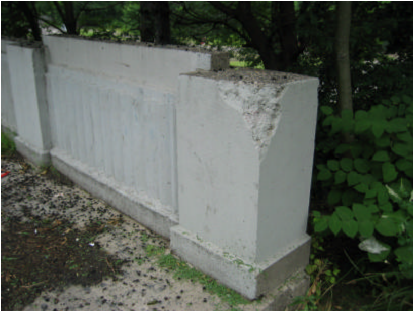
Photo 151 Spalling concrete on the end post of the north parapet wall; note that the wall has been painted to cover graffiti.
