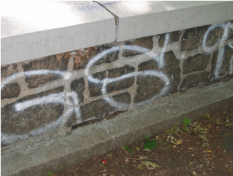
Photo 42 Detail of railing on the east side of Subway 2; note the cracking paint and open mortar joints of the railing and coping stones.
