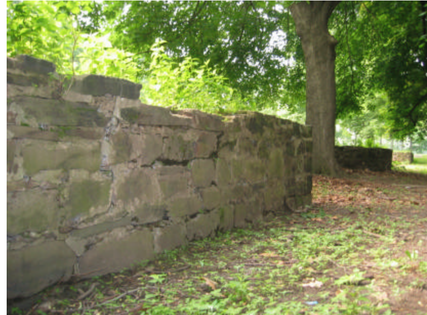
Photo 89 View of wall, stone and mortar details; note the missing coping stones at the top of the wall.
