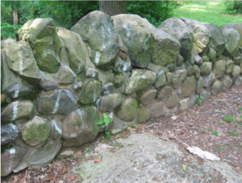
Photo 166 Open and exposed mortar joints at the base of the north cheek wall; note the exposed and eroded top of the concrete arch.
