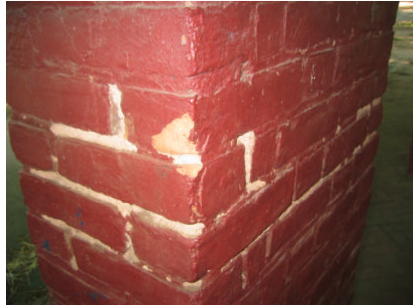
Photo 18 Typical chipping on the corner of the columns.
