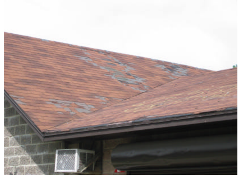
Photo 129 Missing and damaged shingles on the south end of the roof.
