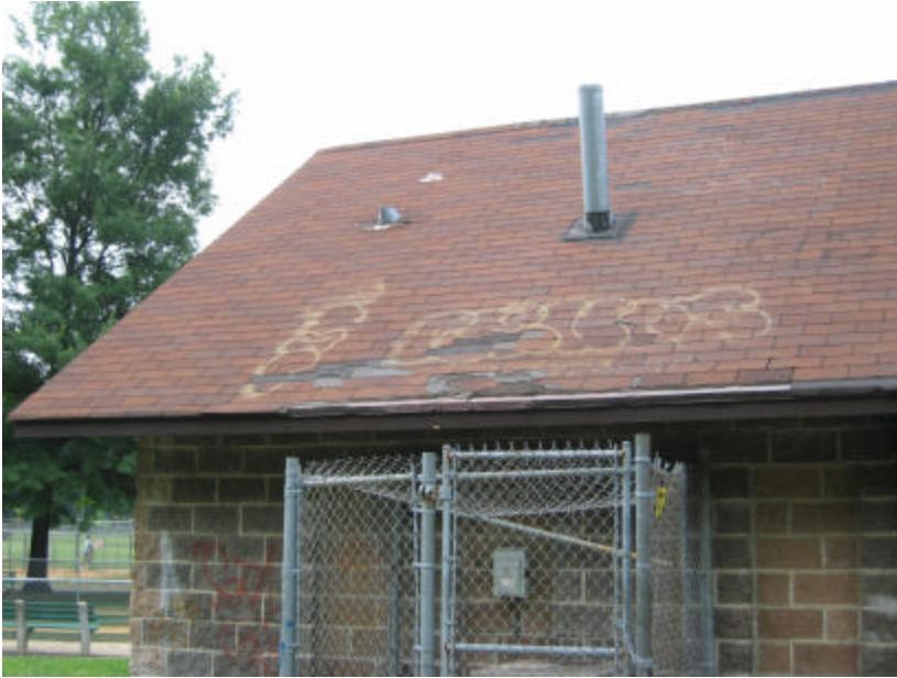
Photo 130 The north slope of the roof has missing asphalt shingles, exposed roof sheathing and graffiti along its edge.
