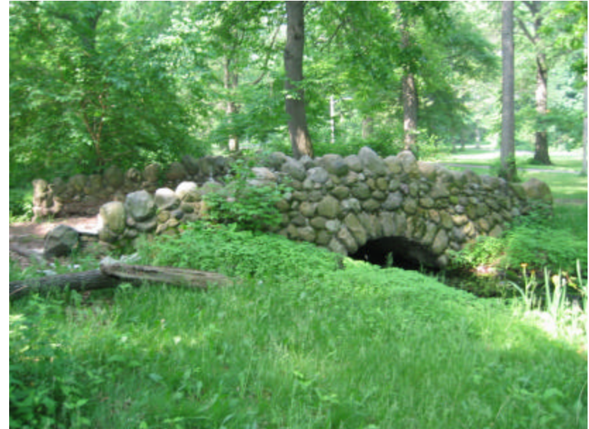
Photo 163 View south towards the footbridge; note the organic growth on the surface of the cheek wall.
