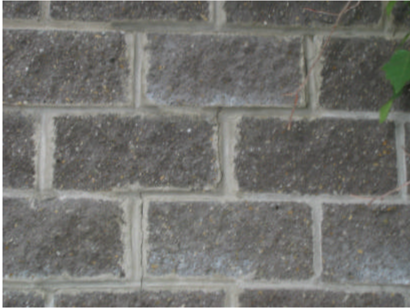
Photo 136 This zigzag crack is approximately 5' – 0" on the west façade of the seniors' building.
