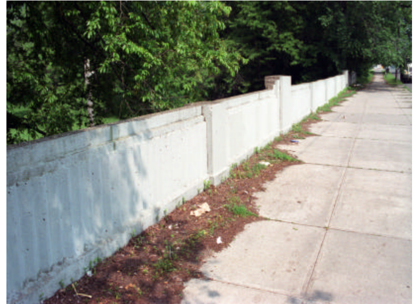
Photo 150 The south parapet wall; note the debris and vegetation along its base.
