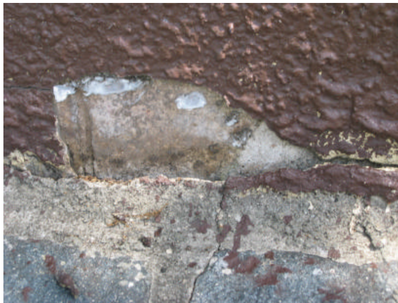
Photo 55 Stucco and mortar that has detached from the base of the north restroom.
