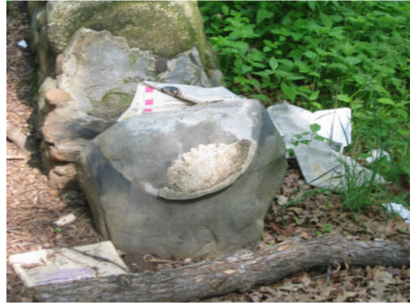
Photo 169 Displaced boulder on the north cheek wall; note the debris around the site.
