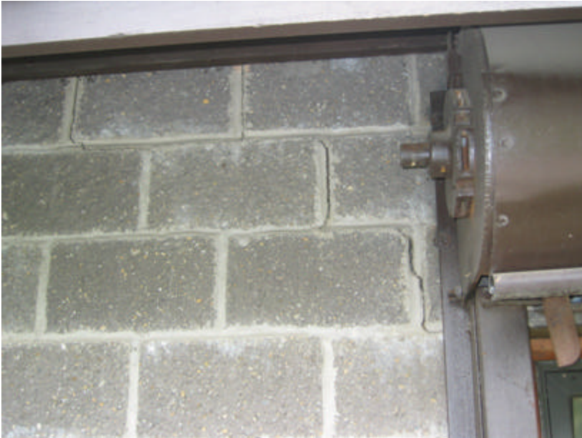
Photo 134 Zigzag cracking from the cornice to a window frame on the south façade of the building.
