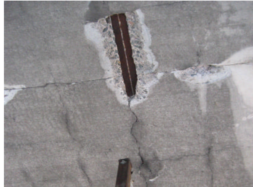
Photo 82 Exposed and rusting section of the Melan arch; note that this may cause severe structural damage to the bridge.
