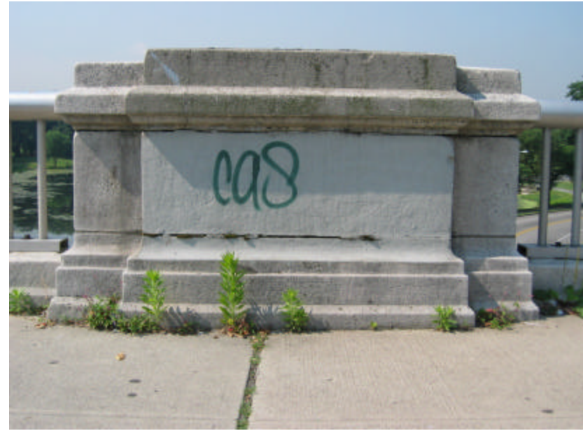
Photo 78 The center railing post on the south side of the bridge; note that it has been patched but still remains in poor condition.
