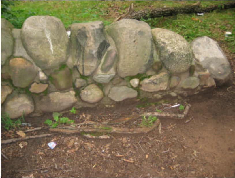
Photo 168 Roots at the base of the north cheek wall; note that they may be damaging the footbridge.
