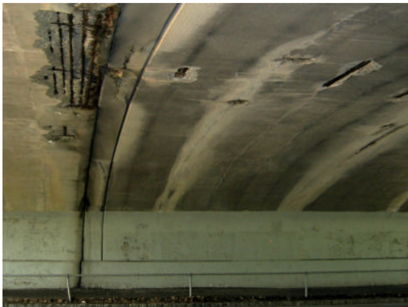
Photo 147 Extreme spalling, cracking, soiling and rusting on the underside of the bridge; note that this damage has occurred where the two arches were joined together during the 1951-1953 renovation.
