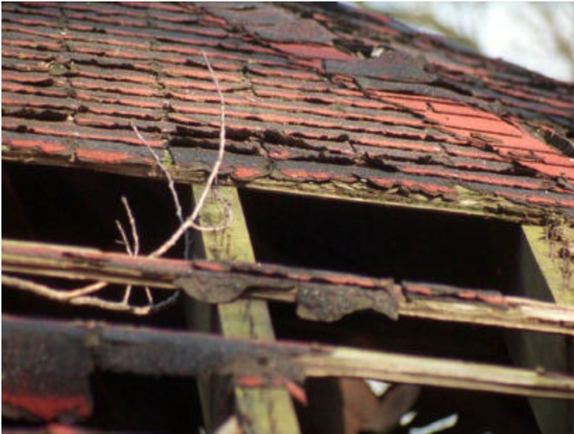
Photo 108 Detail of The Octagon Shelter showing missing wood roof sheathing and failed asphalt shingle roofing.
