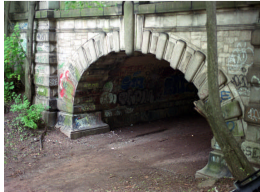
Photo 25 Subway 1, view looking east; note the graffiti and biological growth.
