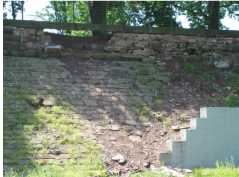
Photo 3 A large hole in the old reservoir wall surrounding the roller rink.
