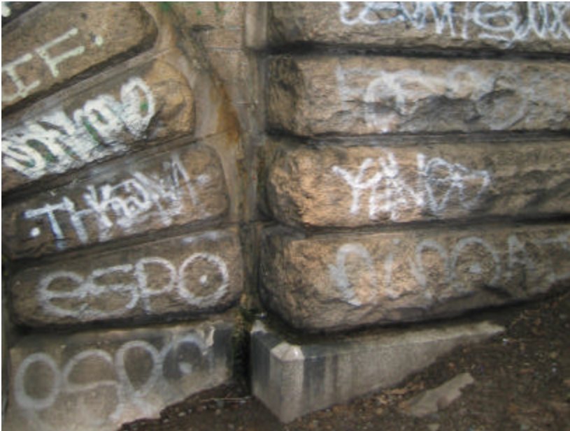
Photo 36 Stonework on the east side, archway and buttress; note the discoloration of the stone.
