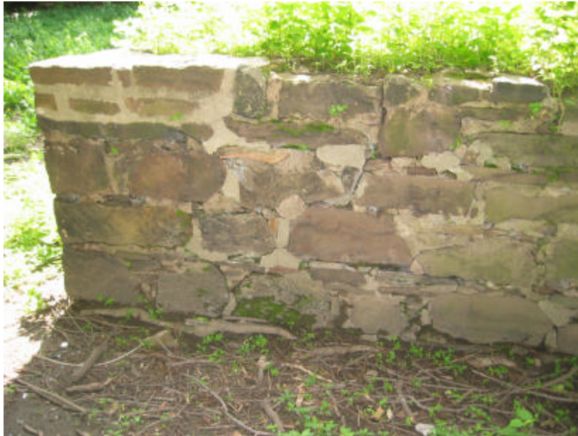
Photo 90 Erosion around the base of the wall; note that the stones at the top of the wall are typically smaller than at the bottom.
