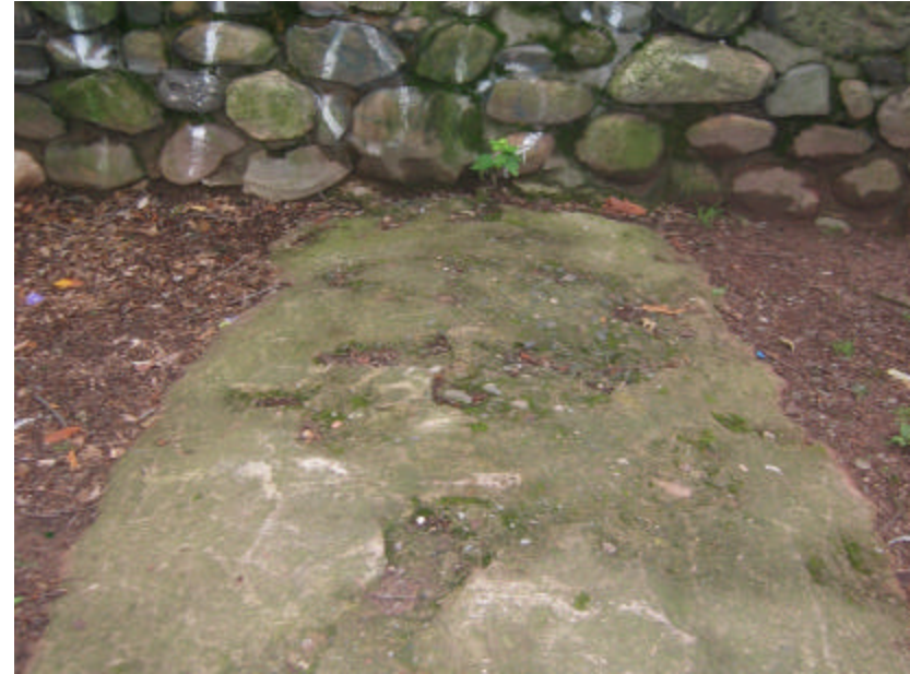
Photo 161 The exposed top of the arched concrete culvert; note the eroded surface exposing aggregate.
