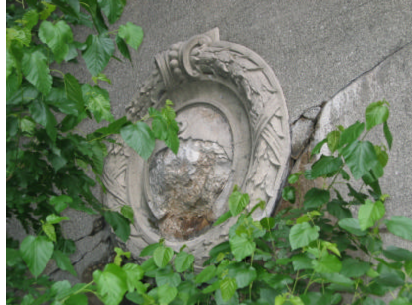
Photo 146 The medallion on the southwest side of the bridge; note that the surface has spalled and the cheek wall is cracking.
