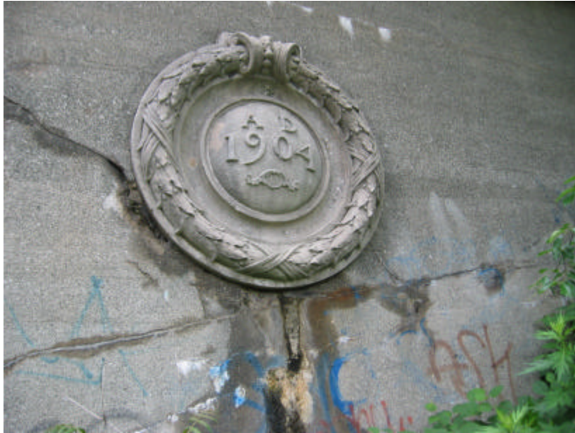
Photo 145 The medallion on the southeast side of the bridge; note the graffiti and the moisture-saturated concrete.
