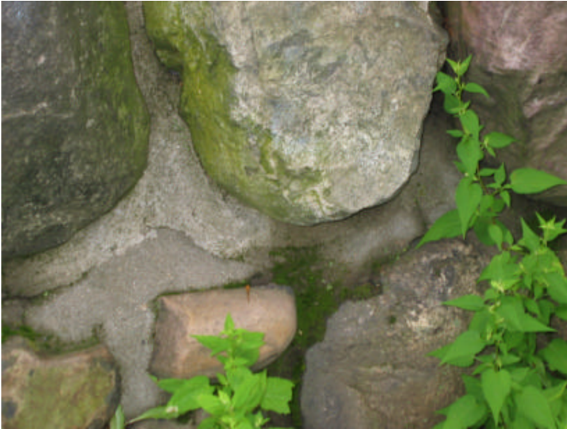
Photo 176 Remedial patching of the mortar joints; note that this joint was not raked back and new mortar was added on top of the old.
