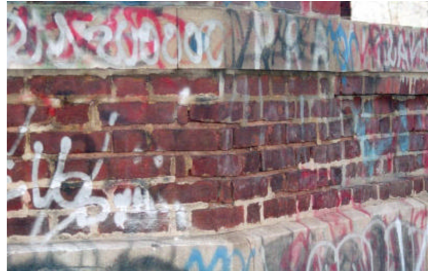
Photo115 Detail of The Octagon Shelter showing typical brick low wall with eroded mortar joints, selective repointing with non-matching mortar and graffiti; note that the original mortar joints are tinted similar to the brick color.
