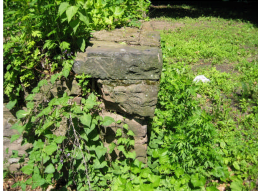
Photo 93 Plant growth coming from a cracked corner of the wall.
