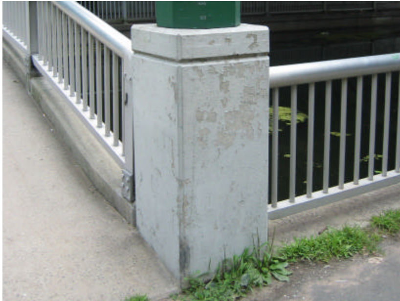
Photo 85 Peeling paint on the concrete posts.
