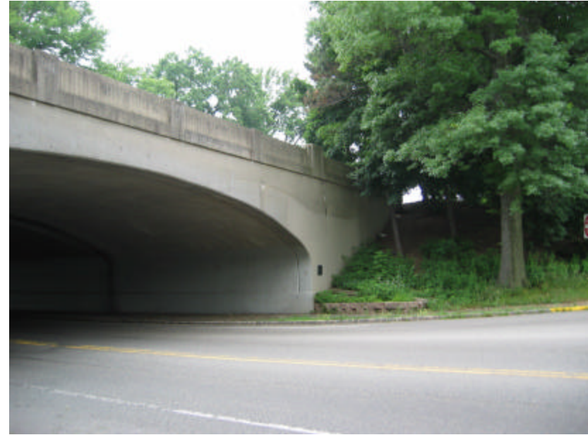
Photo 154 The north side of the bridge; note the soiled top parapet wall and the painted areas of the spandrel and wing walls.
