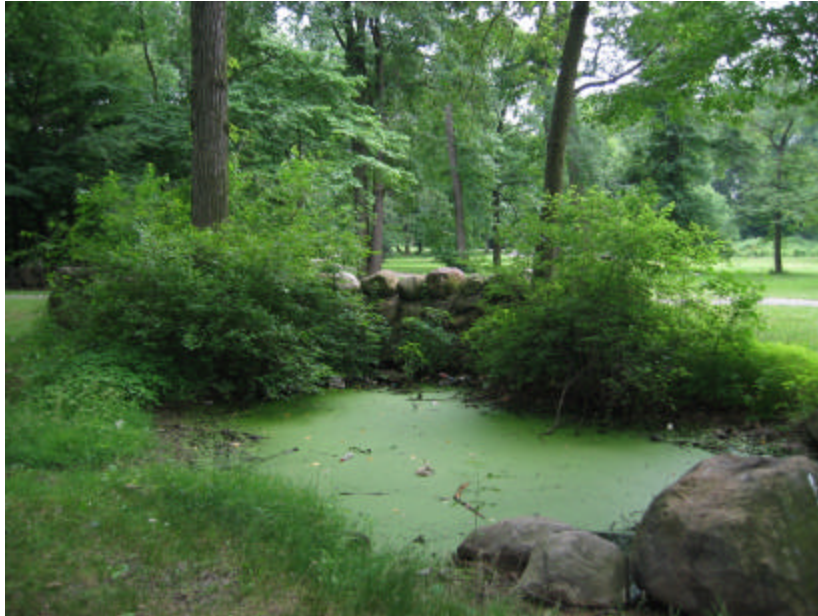
Photo 172 Bushes have overgrown the north cheek wall; note the silting up of the stream has clogged the culvert.
