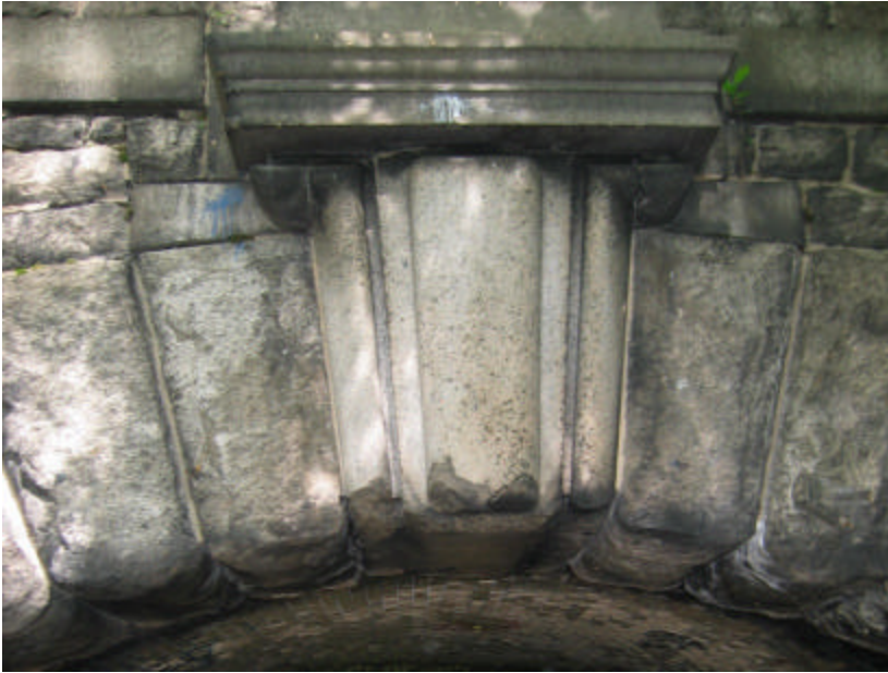
Photo 44 The keystone on the west side of the underpass; note the spalled granite on its base as well as on the other blocks.
