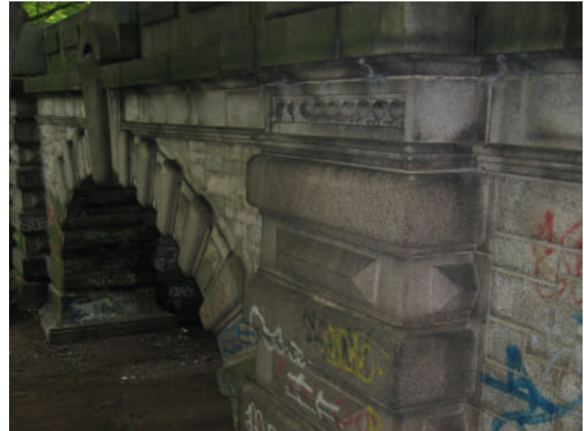
Photo 31 Close-up of one of the buttresses on the west side of Subway 1; note the soiling of the stone surface.
