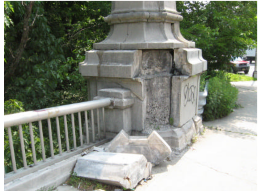
Photo 72 The top of the northeast butters and base of the lamppost; note the large amounts of material that have detached.
