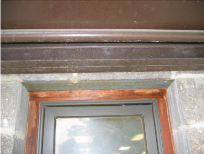
Photo 132 The rusting steel lintel spanning the window opening; note the weathering of the wood window frame.
