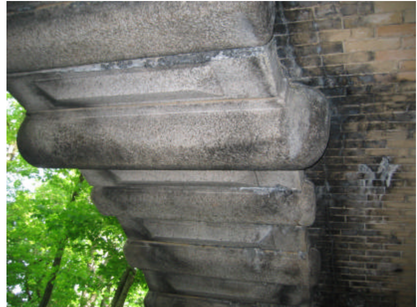
Photo 29 Detail of the alternating large projecting bush-hammered granite blocks and smaller, dressed and beveled granite blocks on the west side of the archway; note the efflorescence on the stones and bricks.
