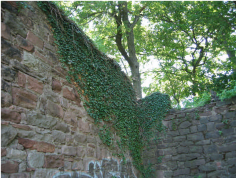
Photo 98 Stones missing from the parapet; note that smaller coping stones are also missing and that ivy is overgrowing a large section of the wall.
