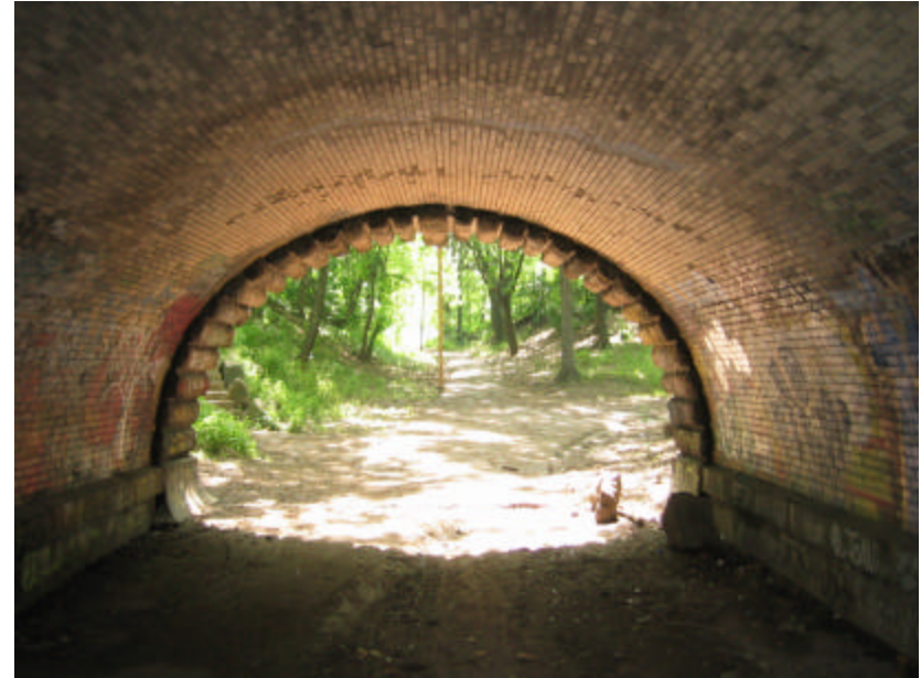
Photo 27 The underside of Subway 1; note the barrel vault construction of the underpass and the debris on the floor of the underpass.
