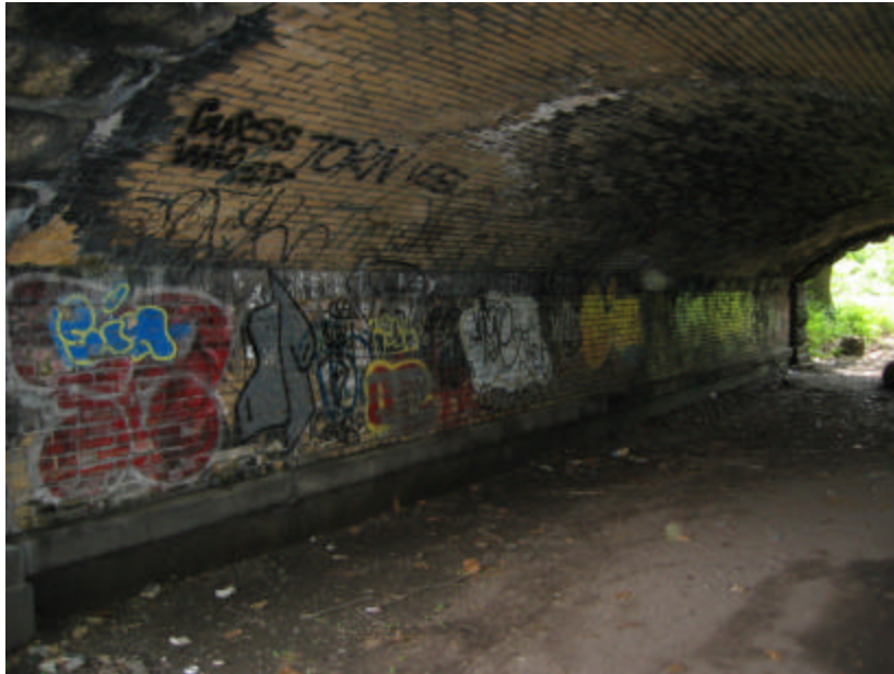
Photo 40 Interior of Subway 2; note the dirt floor and the excessive amount of graffiti and efflorescence.
