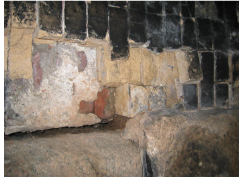
Photo 49 The bricks are so loose in some places that one can pull them out of the vault.
