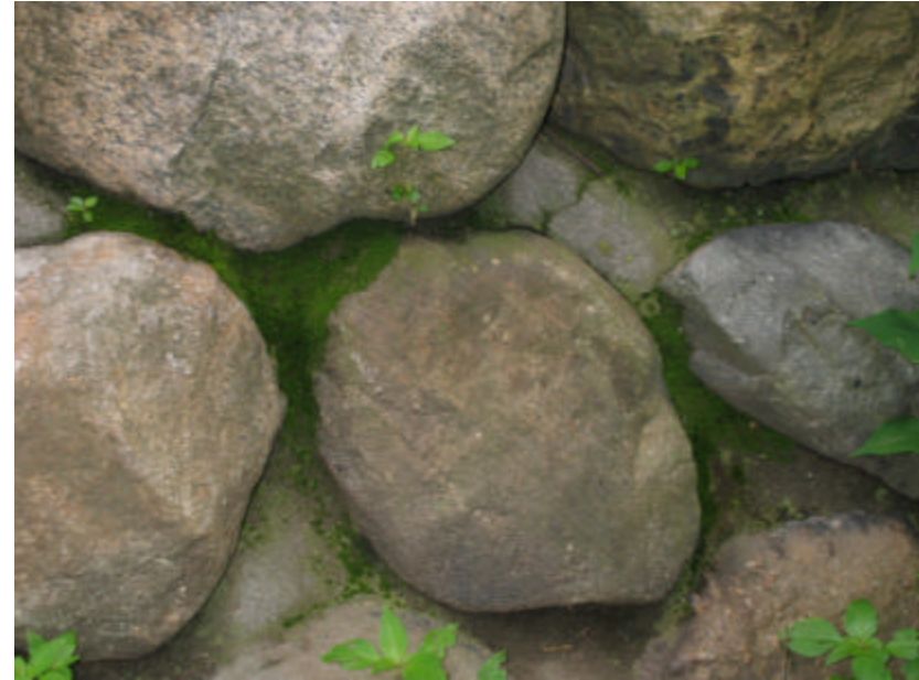
Photo 177 Organic growth including moss and weeds growing from cracks in the mortar.
