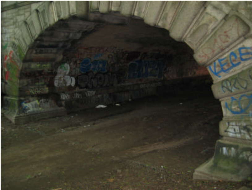
Photo 28 Arched opening of the west side of Subway 1; note the segmental arch construction and soiled, graffiti-covered granite.
