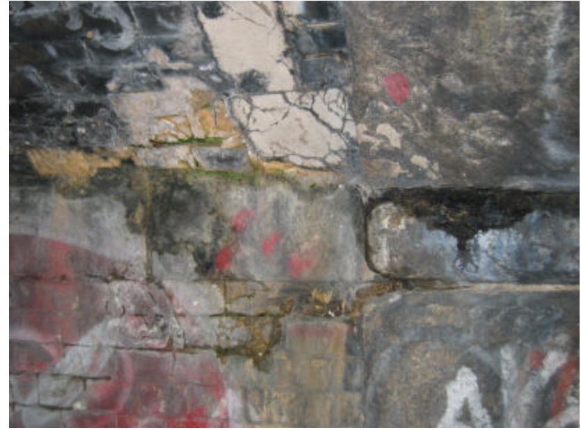
Photo 45 The arch rising from the spring course; note the cracked mortar patching and the black staining of biological growth.
