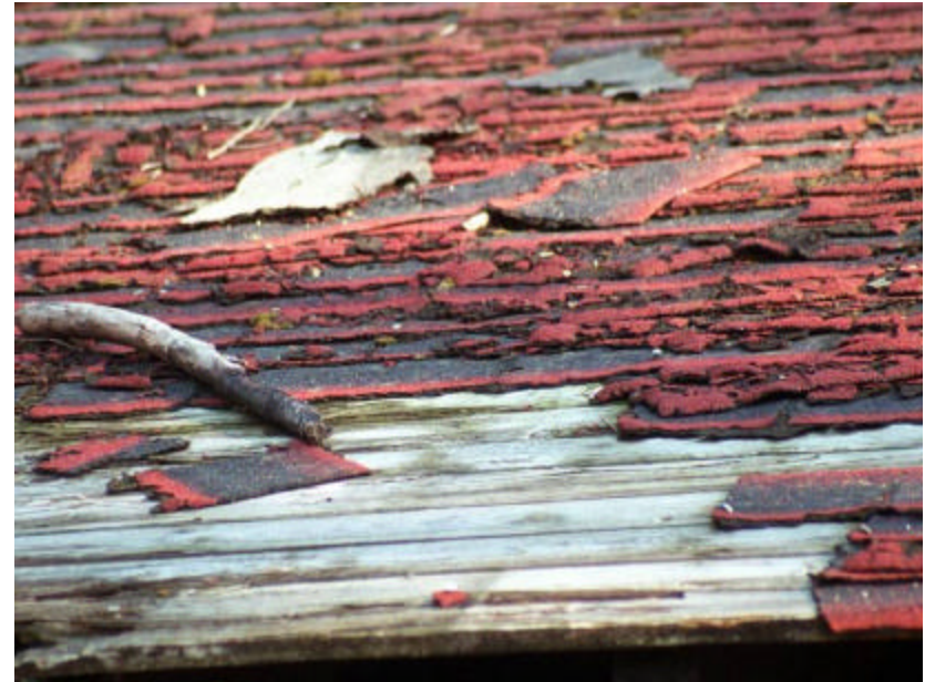
Photo 109 Detail of The Octagon Shelter showing failed asphalt shingle roofing and exposed wood roof sheathing.
