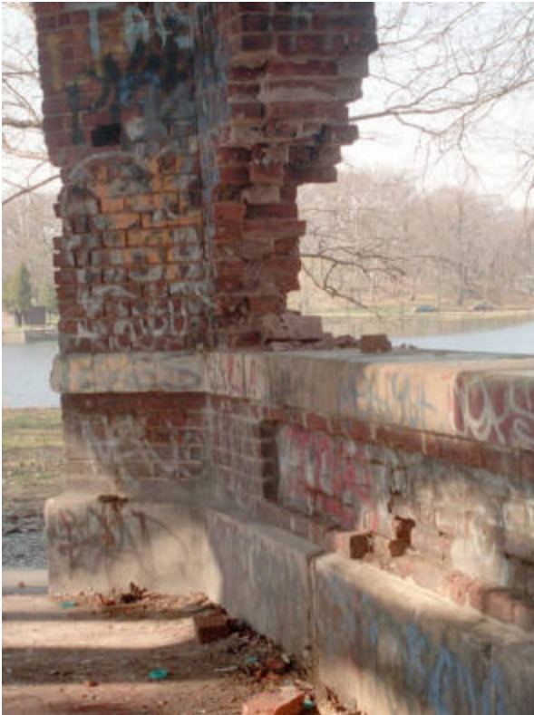
Photo 110 Detail of The Octagon Shelter showing missing brick at column 1.5; note that all masonry surfaces are covered with graffiti.
