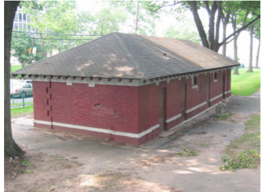
Photo 58 View looking south with Clifton Avenue on the left; note the damage to the north wall.
