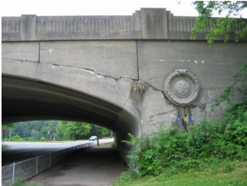
Photo 143 The south side of the bridge; note the vertical and horizontal cracking and spalling.
