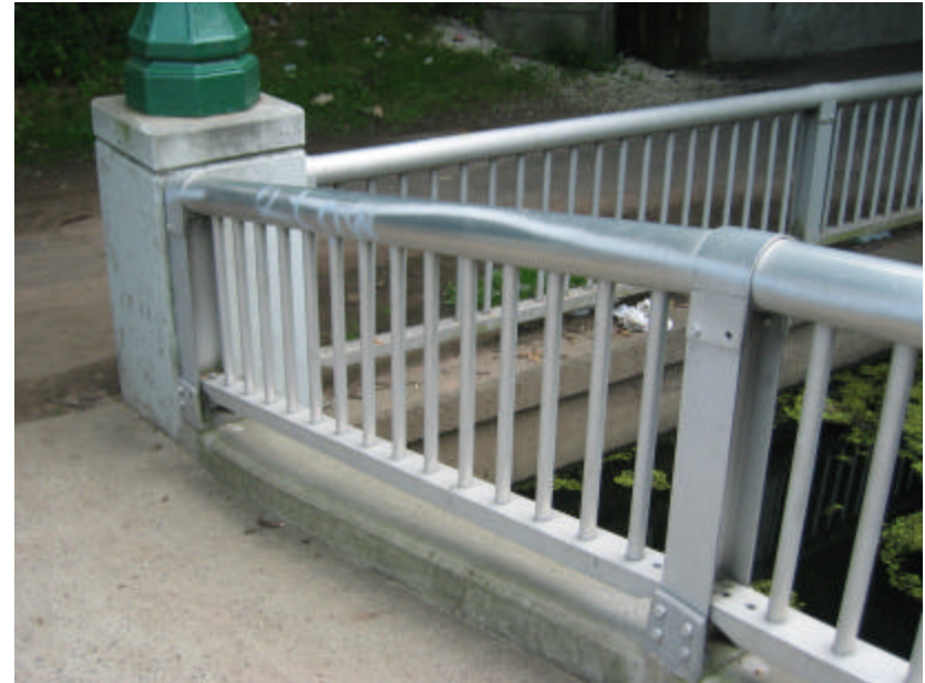
Photo 86 A concrete post at the north end of the footbridge; note the A section of the aluminum railing that is covered with graffiti. A concrete post at the north end of the footbridge; note that the aluminum railing is in good condition overall, but sections are covered with graffiti.
