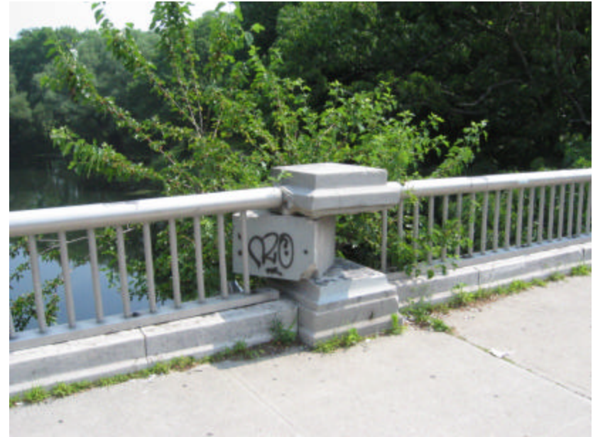
Photo 76 Displaced concrete post in the balustrade; note that this is an extremely dangerous situation since this block could fall, causing a fatal injury.
