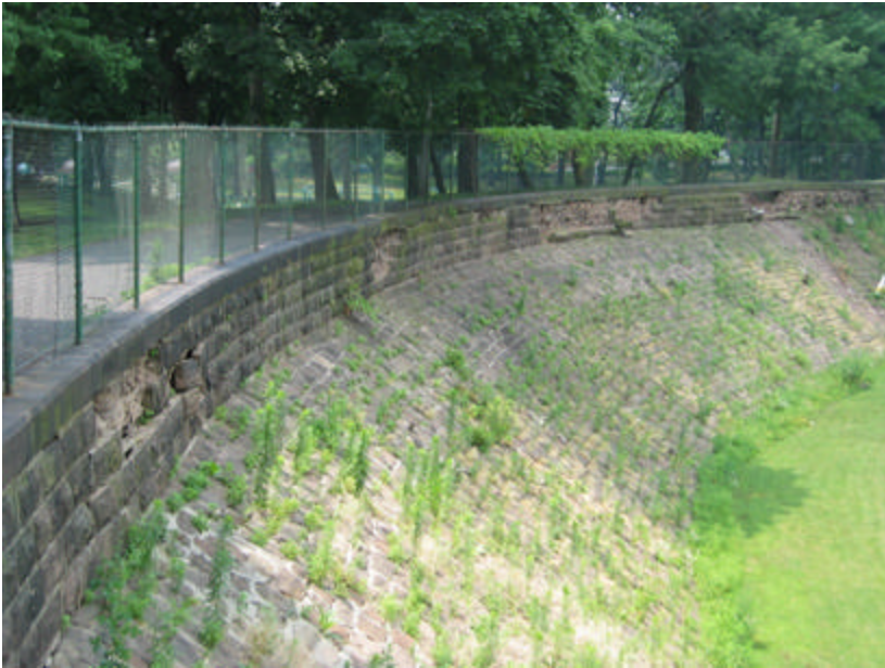
Photo 6 Areas of spalled and missing stone along the wall at the top of the reservoir; note that some areas of spalled brownstone are over 40' – 0" in length.
