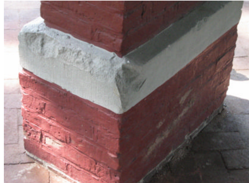
Photo 16 Significant chipping and wear to one of the limestone base caps.
