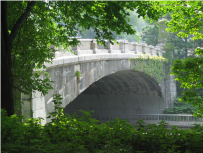
Photo 67 The Park Avenue Bridge from the southwest embankment; note the soiled and fractured face of the arch.
