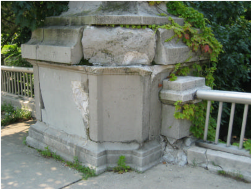
Photo 73 The effects of freeze-thaw cycles on the top of the southeast buttress; note how many of the joints are open and exposed.
