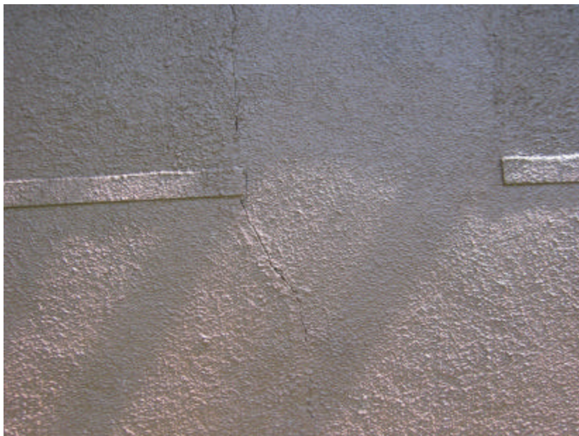
Photo 54 A full height crack in the south wall of the north restroom.
