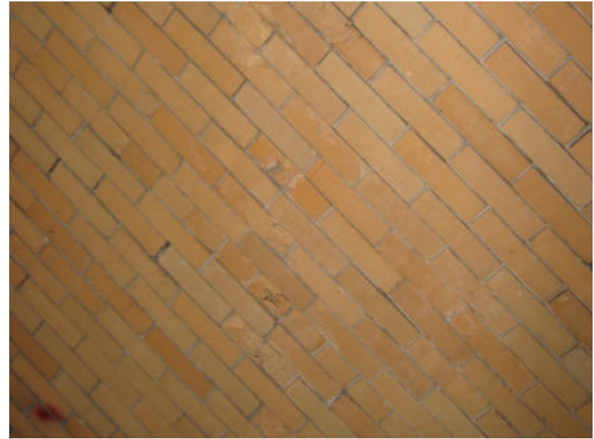
Photo 37 The effects of freeze-thaw on bricks; note the face of some bricks has spalled off and there is loose or missing mortar around most of the brick joints.
