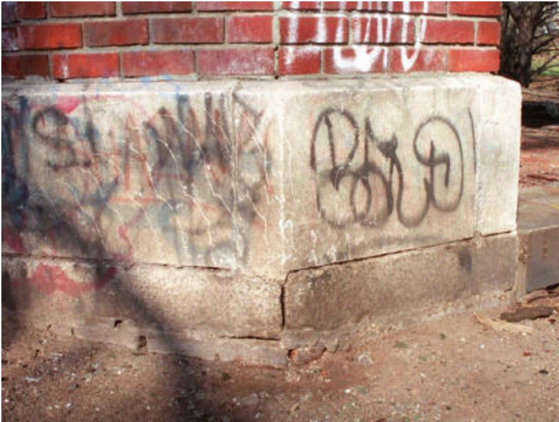
Photo 114 Detail of The Octagon Shelter, column No. 5.5 limestone base with brick foundation exposed by soil erosion, under granite plinth; note that the open corner joint indicates some differential settlement.
