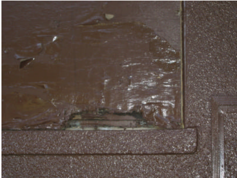
Photo 52 One of the windows that is boarded up on the north restroom; note the plywood covering has rotted because of water damage.
