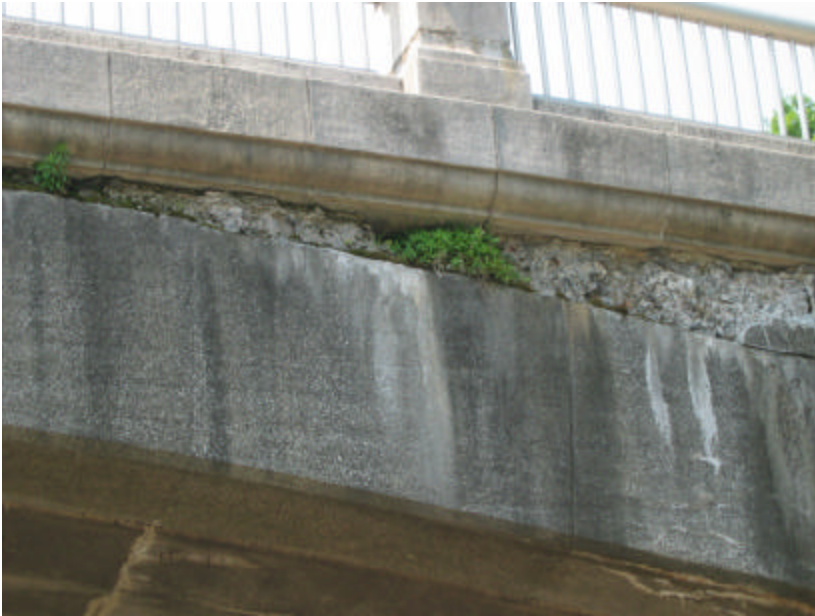
Photo 81 The face of the south arch of the bridge directly below the railing; note that this area of spalling is approximately 10' - 0" long.
